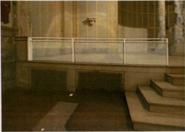
RAISED FLOOR EDGE RAIL DETAIL TIE NEW RAILING INTO REMENENT OF HISTORIC RAILING WITH SIMPLE MODERN STEEL RAILING WITH GLASS INFILLING BETWEEN
