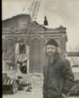
Holy Rosary's Father Metzger at the rear of the former school as it is demolished Source: Columbus Metropolitan Library
